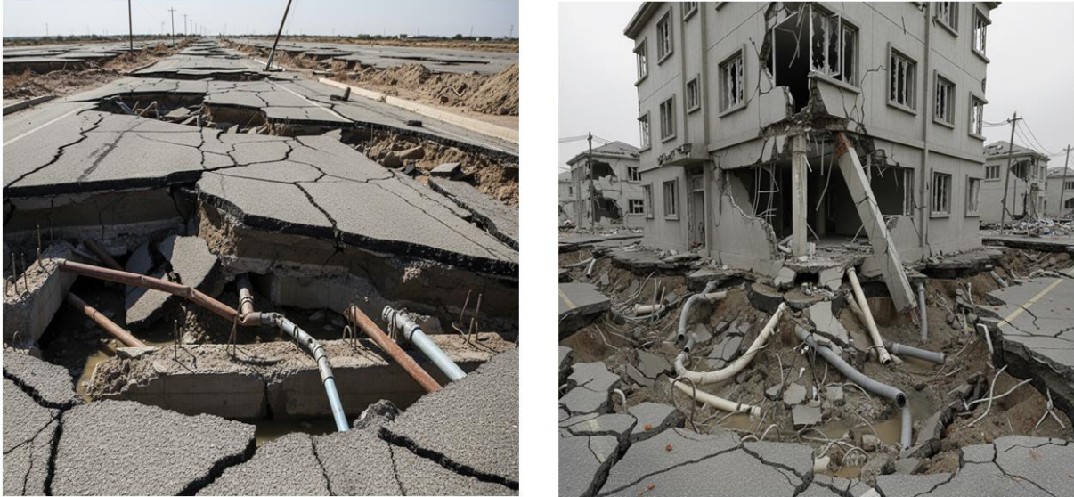
Figure 1.4: Examples of structural damage caused by swelling soils. [8]
